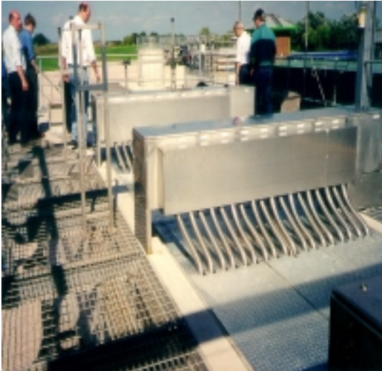
Fig 6 Southport WwTW UV plant
