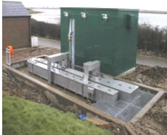
Fig 7 Preesall WwTW UV plant
