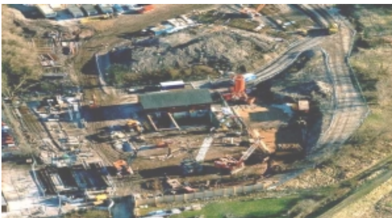
Fig 5 Lytham PS and storage tank
